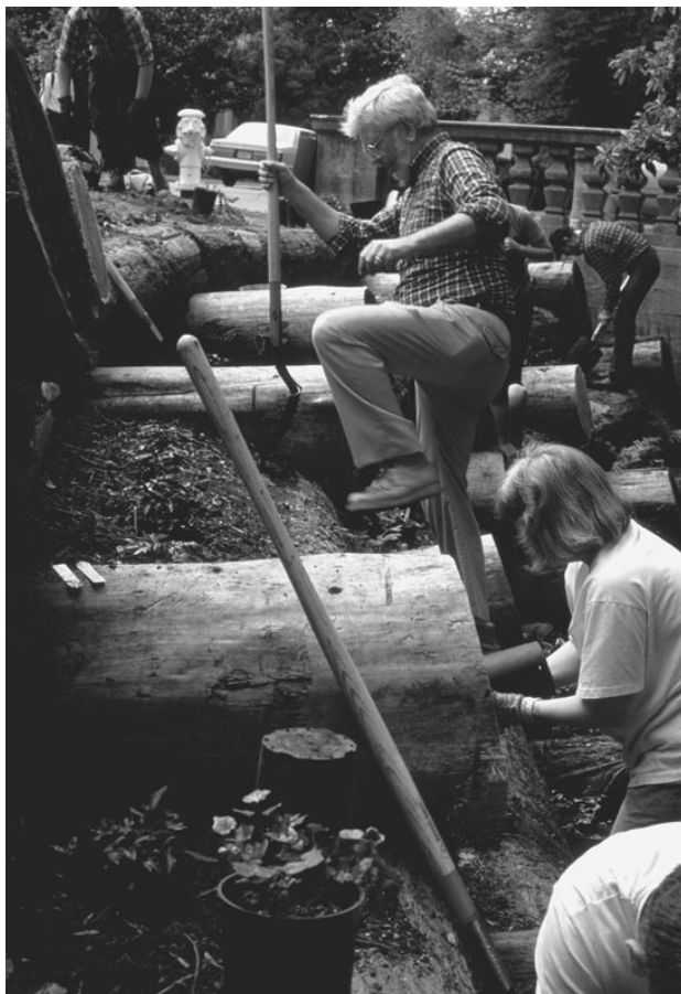
Planting crib walls on Strawberry Creek, at the University of California Berkeley Campus.
