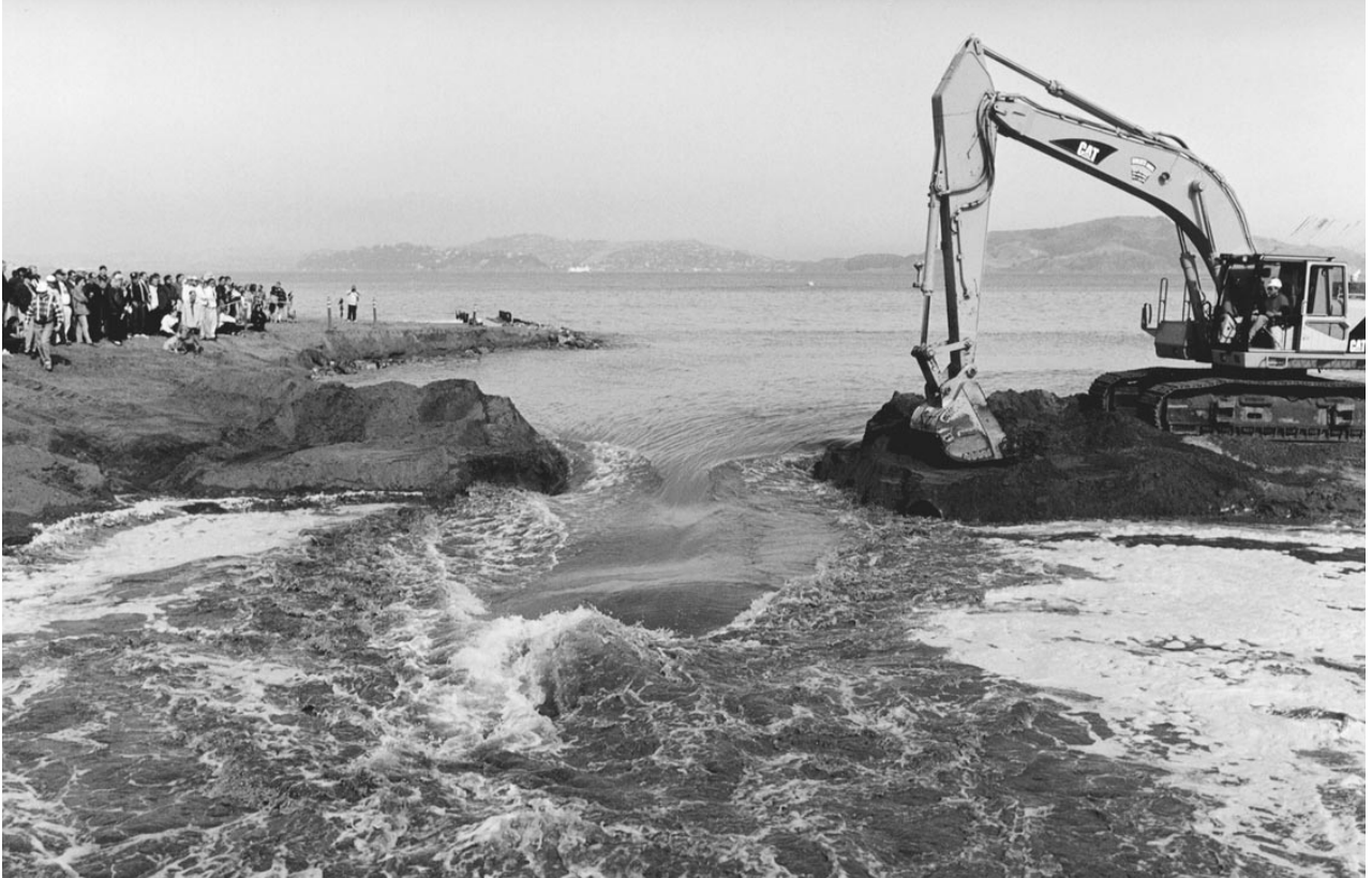
This levee was breached to reopen a tidal wetland at San Francisco's Crissy Field (November 1999).
